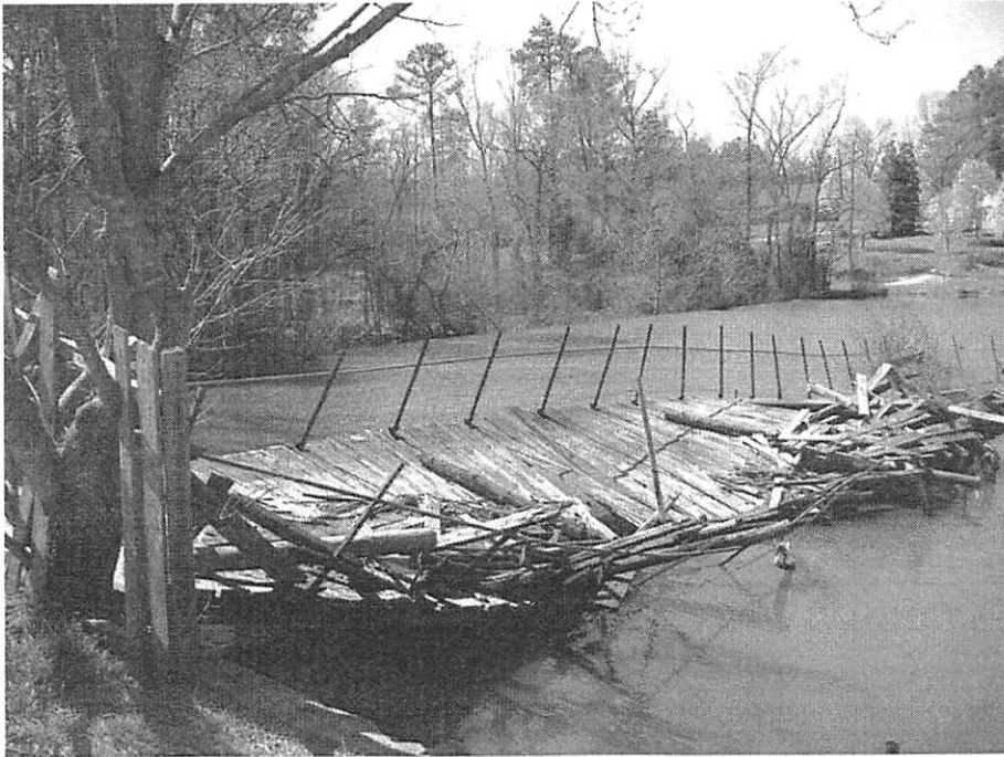
Figure 17: The collapsed boardwalk and dock at Lake Myra in 2008. In the past, visitors to Lake Myra would have been able to fish and swim off of the boardwalk.
