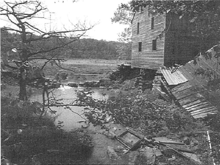
Figure 9: Yates Mill after Hurricane Fran. Notice that the shed attached to the mill has collapsed, and that the original dam was destroyed. It is believed that the dam had stood since its construction in the mid 1700s. Photo taken by Rebecca Cope; courtesy of Historic Yates Mill County Park.
